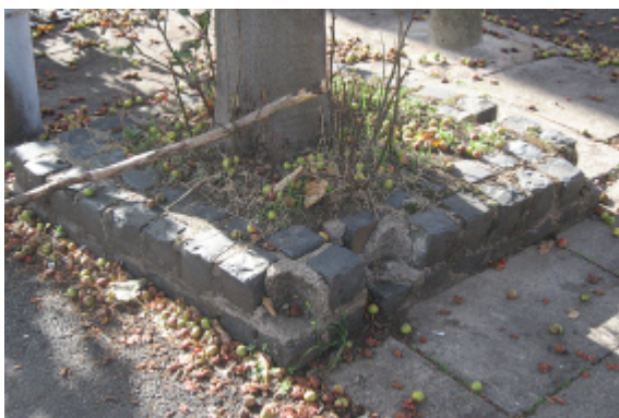
Dilapidated planter Park Street.
