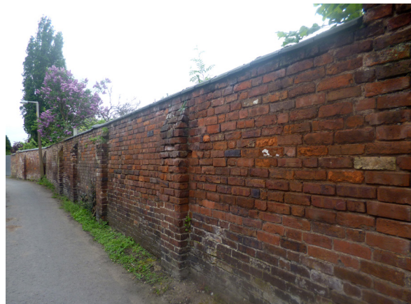
A brick wall enclosing plots from the back lane, St. George's Lane South
