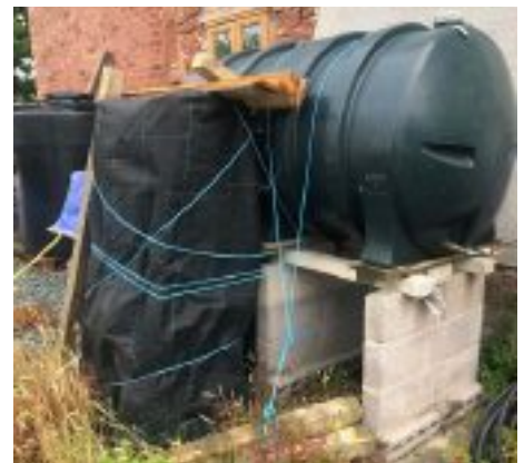
Oil tank housed and secured above highest flood level.
