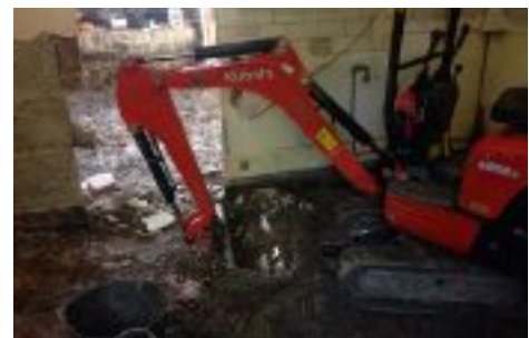
The rebuild involved excavating and 'tanking' the whole of the ground floor
