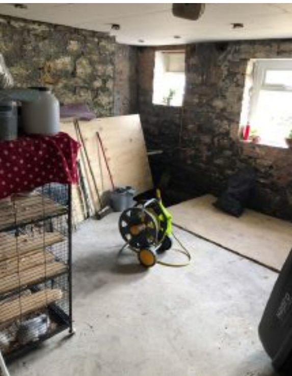
The basement room previously housed the kitchen and was extensively flooded to a depth of 5 feet.
