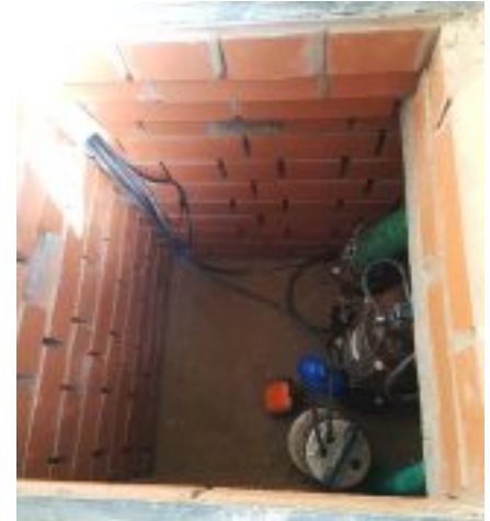
Two sump-pumps in lounge.
