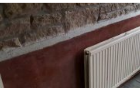
The walls were rendered on top of the membrane, using coloured renders
