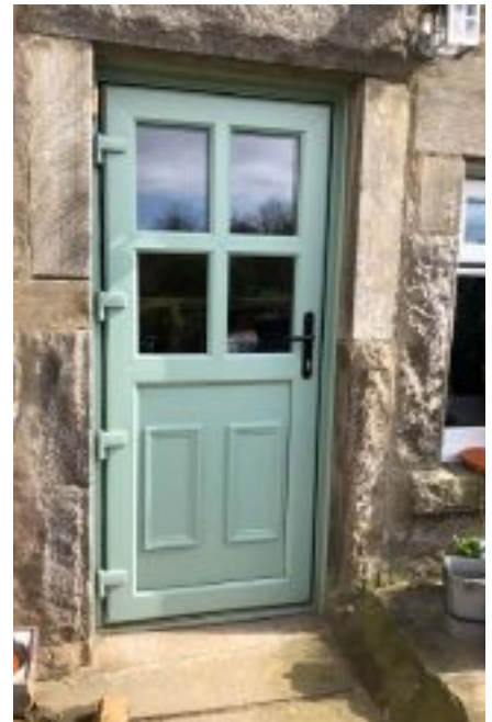
Flood door fitted.
