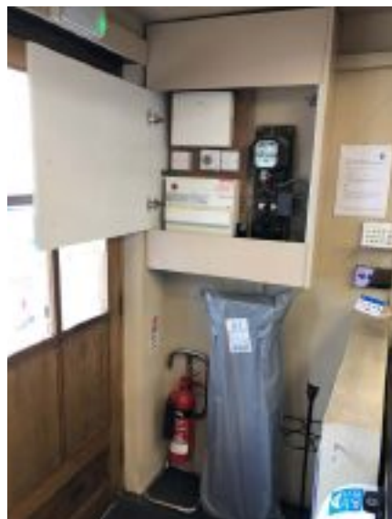
Electric meter and fuse box sited high up.
