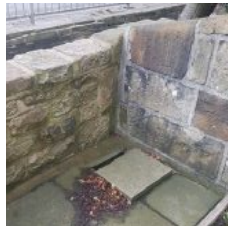
Sump created, into which powerful submersible pump can be dropped when flooding commences.
