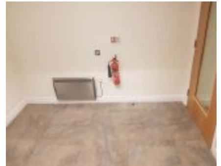
The lower section of the wall was re-plastered using a breathable renovating plaster.
