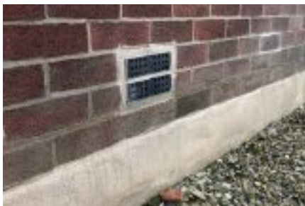
Self-closing air bricks and waterproof rendering was applied underground to the foundations and 30cm (12") above ground.
