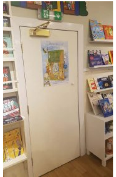
Plastic door architraves.
