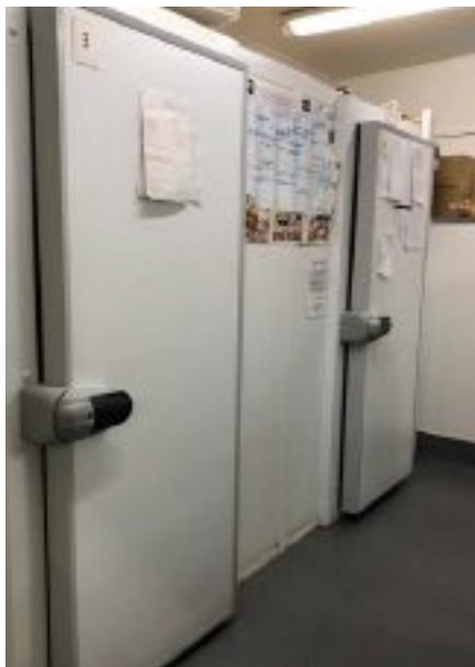
Cold stores have fitted rubber seals but in addition marine ply is sealed to the fronts.
