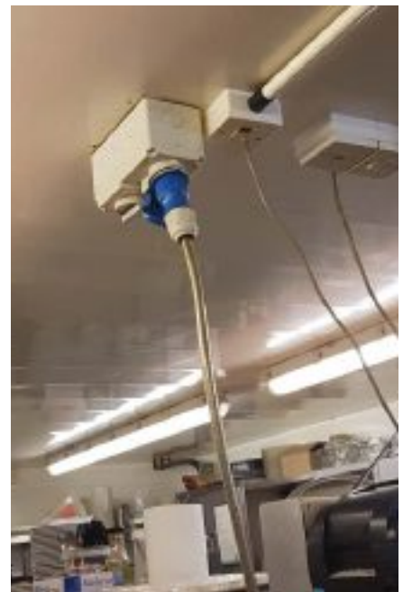
The electricity and gas supply are high up and can be easily turned off and back on.
