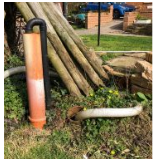
Rainwater runs through a series of French drains into a large sump into which a strong pump is fitted which pumps the water outside the garden boundaries.
