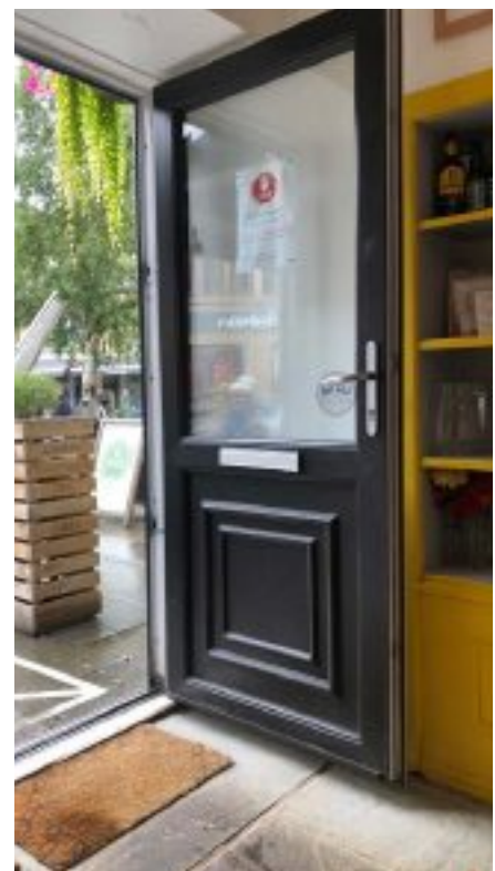
Kitemarked flood door and stone flagged floor.
